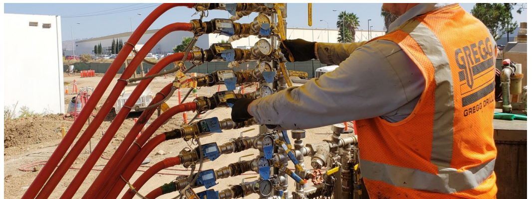
Photo: Gregg Drilling team treats contaminated groundwater under a biomedical lab in California
